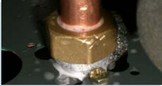
A soap bubble test can detect small leaks
